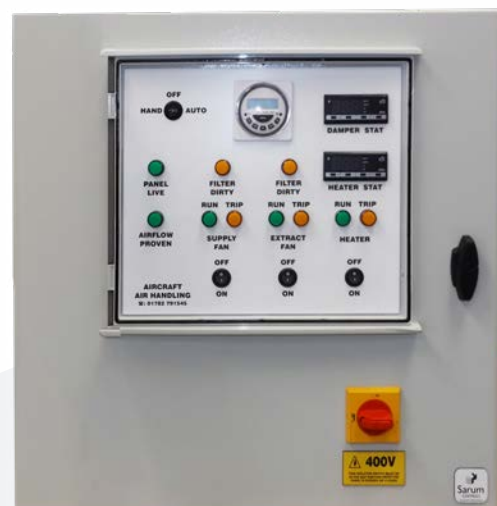
Typical AHU control panel
